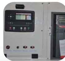
Control Panel & MCB
